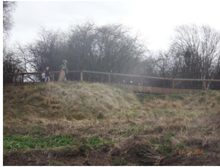
Damaged fencing at Princess Dock-temporary repair carried out by Science Centre personnel
