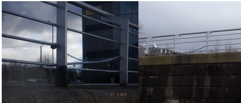
Extension poles for lifebelt poles to enable GPS signage to be above easy reach of vandals
