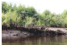
Wooden piles on the south bank between Rutherglen and Smart Bridges are a permanent hazard.
