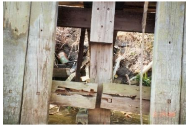
Broken dolphins showing gaps.
